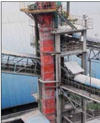
Hoisting conveyor chain for bulk material
