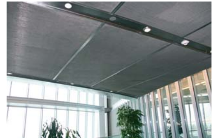
Sede central de ADIA (Abu Dhabi Investment Authority) ADIA Headquarters [Abu Dhabi-EAU]
